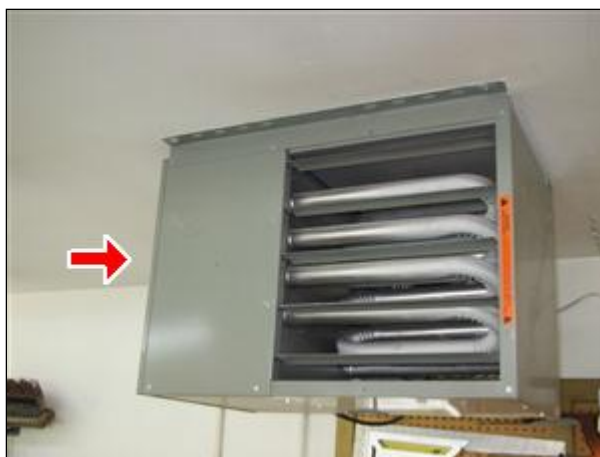
7.11 Picture 1 Gas Furnace in Garage
