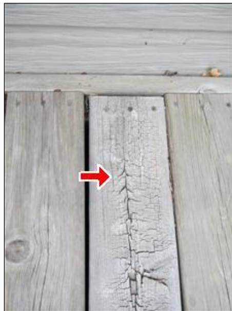
4.3 Picture 1 Warped Deck Board
