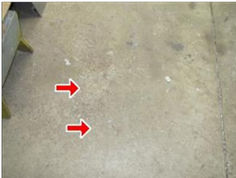
7.6 Picture 1 Spalling On Garage Floor
