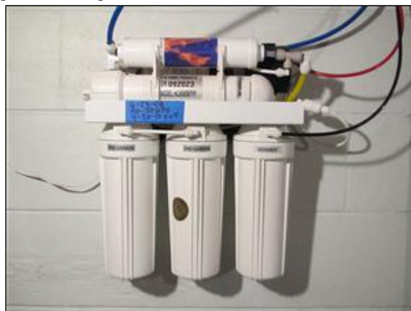
15.6 Picture 1 Reverse Osmosis System
