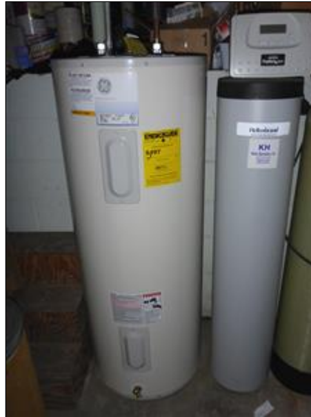
Water Heater And Softener
