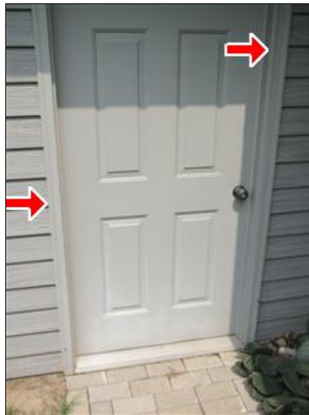
2.2 Picture 1 Paint Service Door Trim
