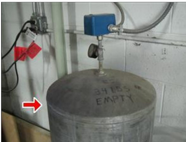
6.0 Picture 1 Pressure Tank
