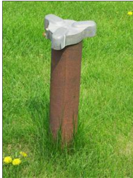
Septic System Vent Pipe
