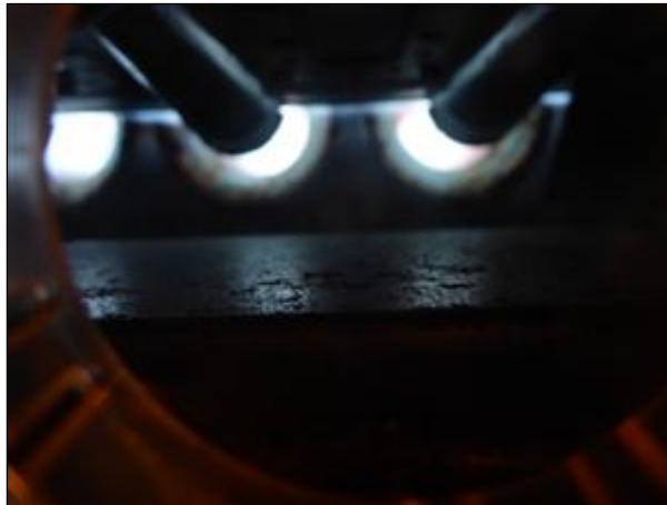
Blue Burner Flames – Good
