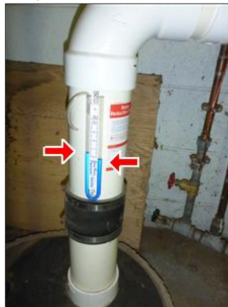
14.12 Picture 2 Vacuum Gauge For Radon System
