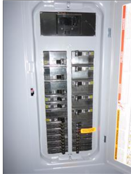
Square D Service Panel
