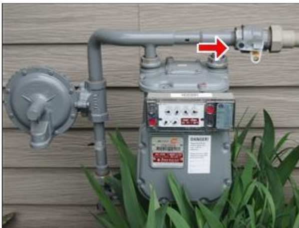
15.7 Picture 1 Main Gas Shutoff Valve
