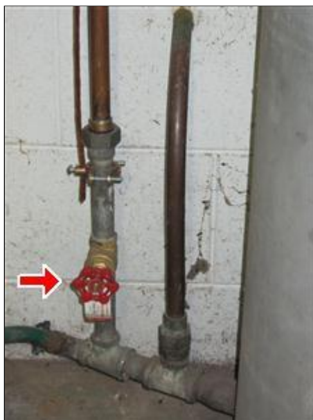
15.8 Picture 1 Main Water Shutoff Valve
