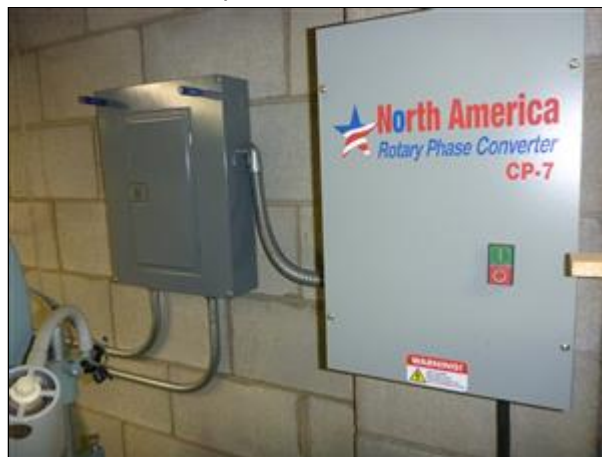
13.8 Picture 1 Three Phase Converter Panel And Distribution Panel
