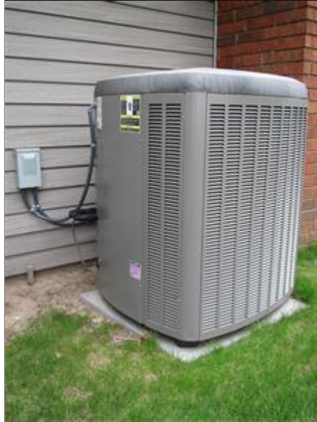
Air Conditioning Condenser
