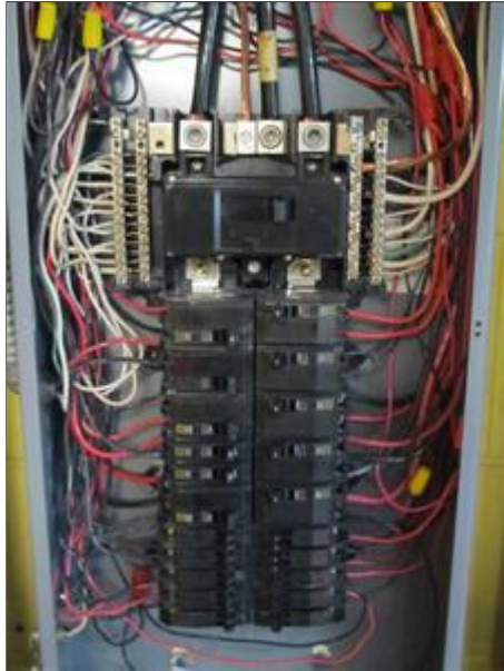
Inside Of Service Panel
